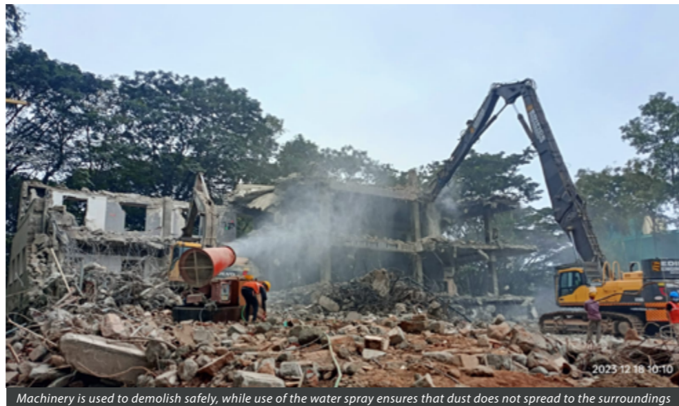
Machinery is used to demolish safely, while use of the water spray ensures that dust does not spread to the surroundings
